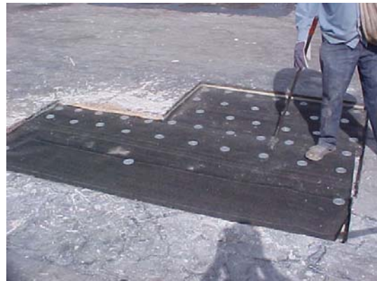
14. Fastening New Base Sheet to Gypsum Concrete After the Concrete Is Set
