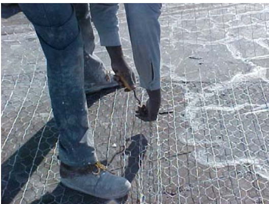
10. Installation of Ties to Connect Old Wire Mesh to New Wire Mesh Around Perimeter of Repair Area
